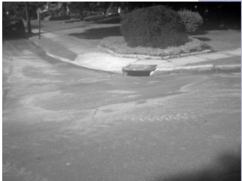
Stormwater that runs through the paved streets of urban and suburban neighbors is collected by dirty, sediment-lined storm drains like this, and is inevitably discharged into local water sources. Photograph courtesy of EPA
