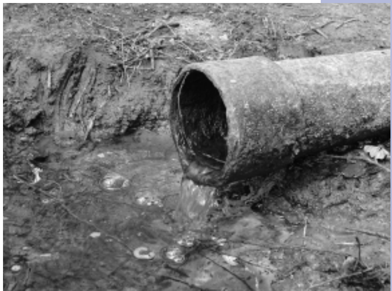
Aging water and sewer lines plague communities in Pennsylvania, costing taxpayers millions of dollars each year.
