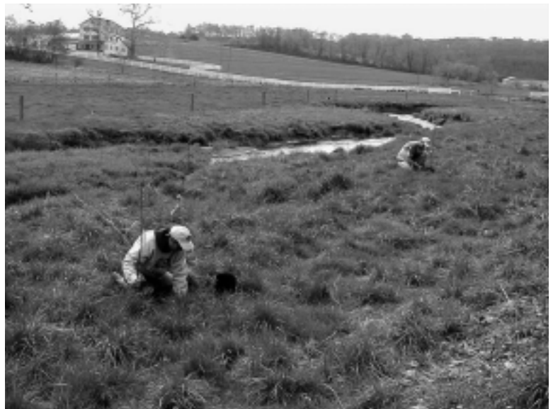
Buffers, like this riparian corridor being planted in Chester County, PA, can serve multiple purposes: reducing runoff and providing recreational space. Photo courtesy of Chester County Water Resources Authority
